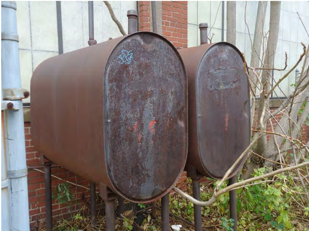
Photograph 12: Fenced-in AST area
