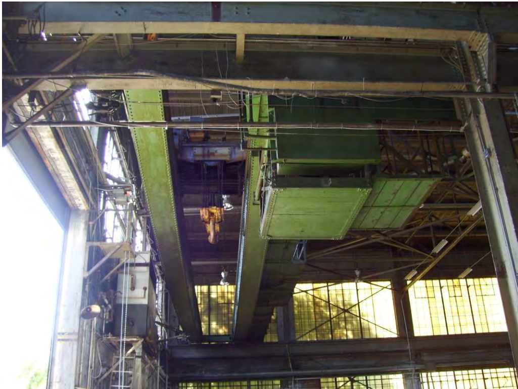
Photograph 4: Crane system (Photograph taken Sept. 2011)
