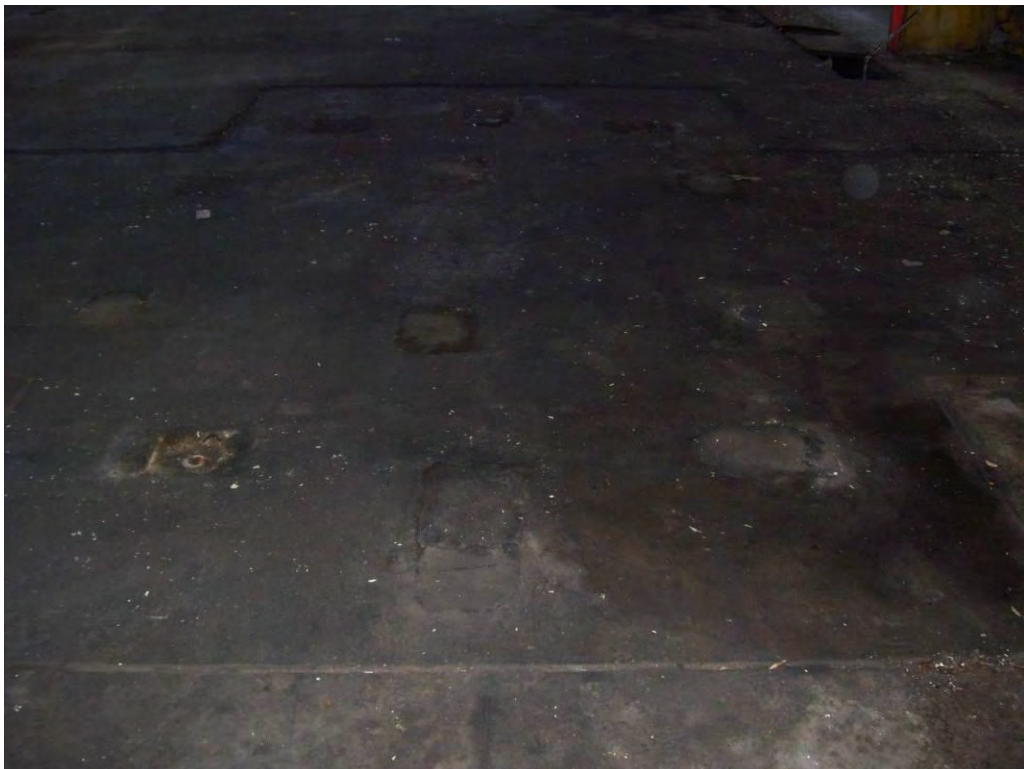
Photograph 2: Possible concrete-sealed floor drains (Photograph taken Sept. 2011)
