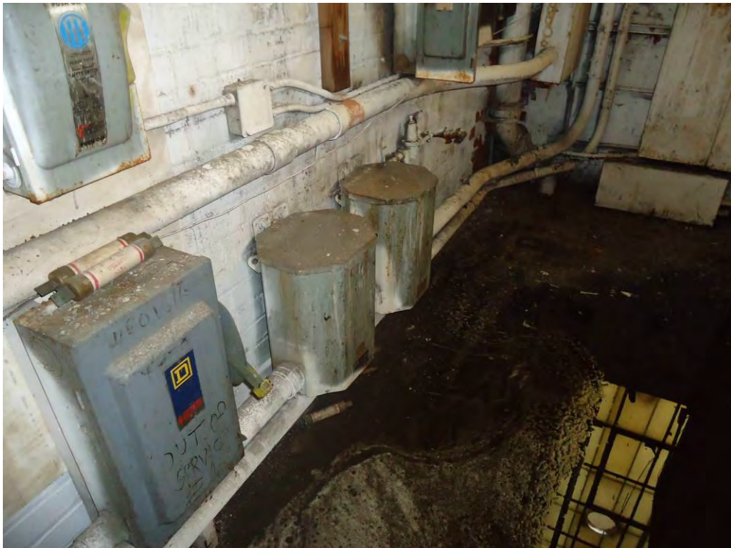
Photograph 6: Suspected PCB-containing electrical transformers
