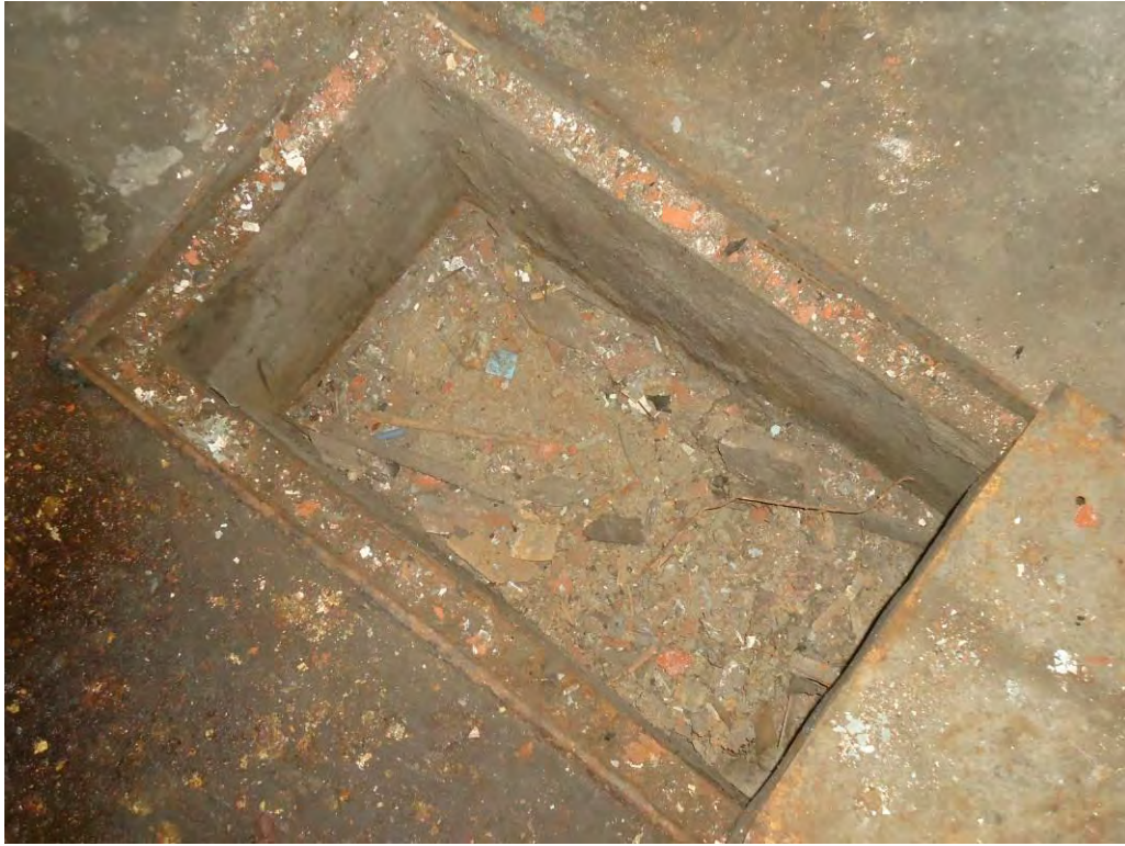
Photograph 3: Open floor trench filled with debris
