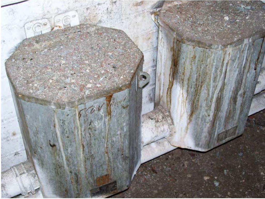
Photograph 7: Two transformers in electric area
