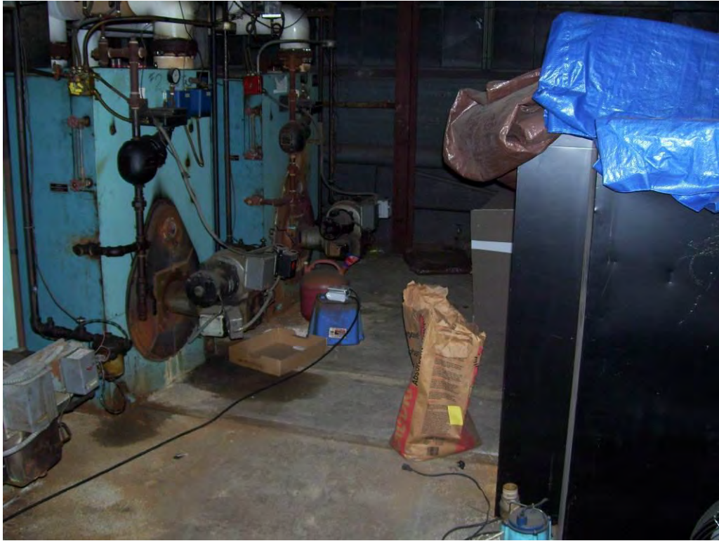
Photograph 5: Boiler room (Photograph taken Sept. 2011)
